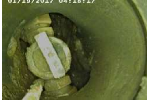
Non-Lead Service Line
