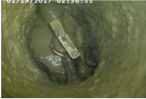
Lead Service Line
