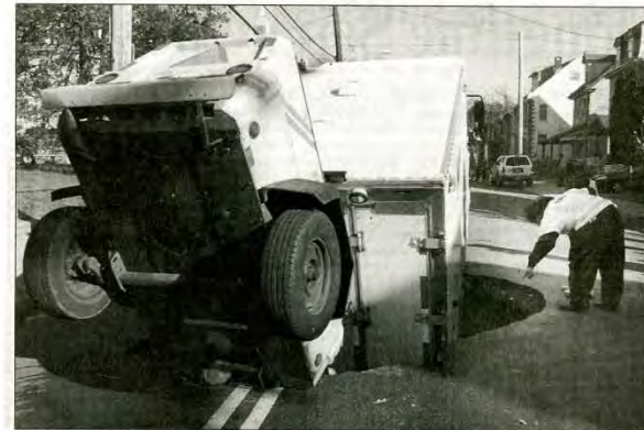
LAURENCE KESTERSON / Staff Photographer A Philadelphia Water Department worker looks at a truck in the Johnson Street sinkhole.
