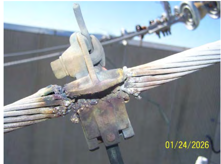
Aerial Electrical Cable
